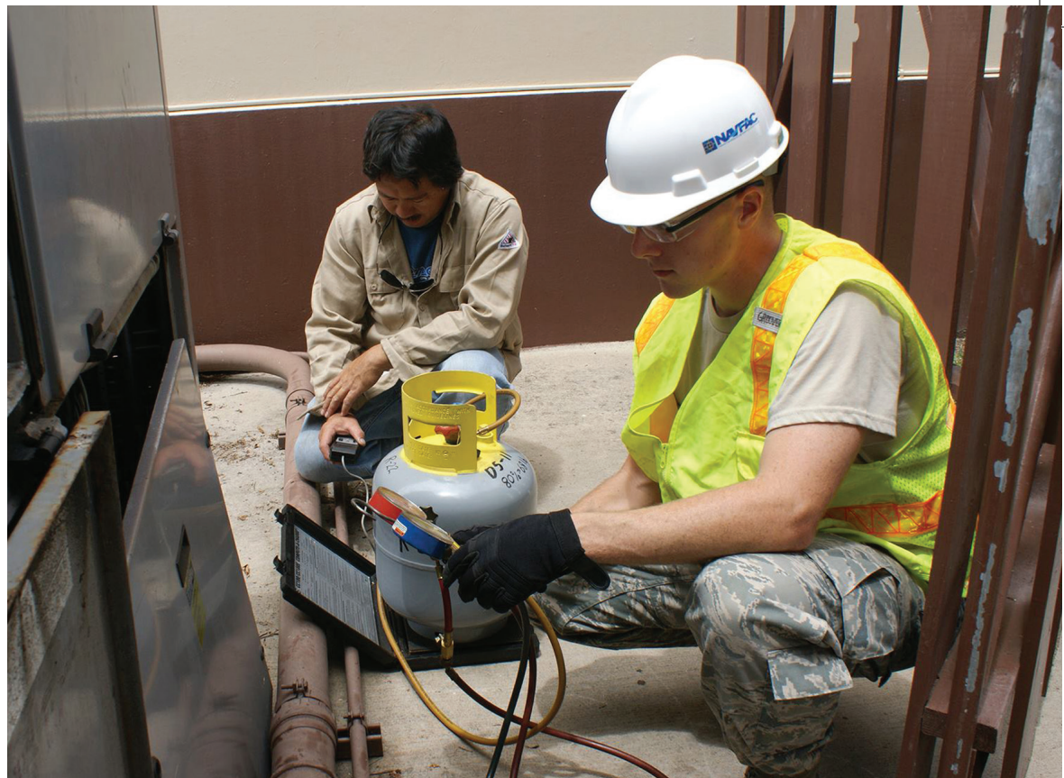
An HVAC professional can inspect and test a furnace to make sure it operates safely and efficiently. PHOTO BY NAVFAC HAWAII HVAC SPECIALISTS
