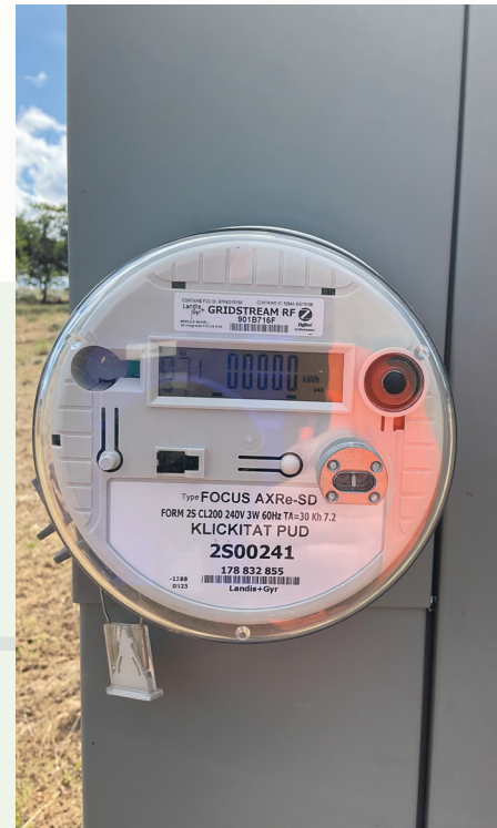
KPUD's newly installed meters provide the utility with real-time updates, allowing KPUD to quickly locate and respond to outages.
