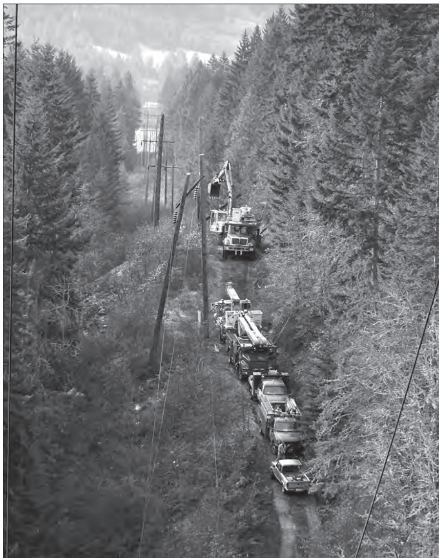
KPUD line crews work on a transmission outage in one of the most remote stretches of line in the county: the Glenwood transmission line.
