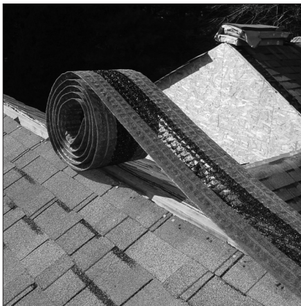
Roll out the ridge vent, smooth it down and cut it to length.
