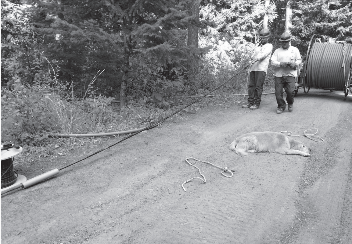
Klickitat PUD linemen Bernie Predeek, left, and Justen Greenwood work around guard dog Stanly as they pull underground wire into a ditch.
