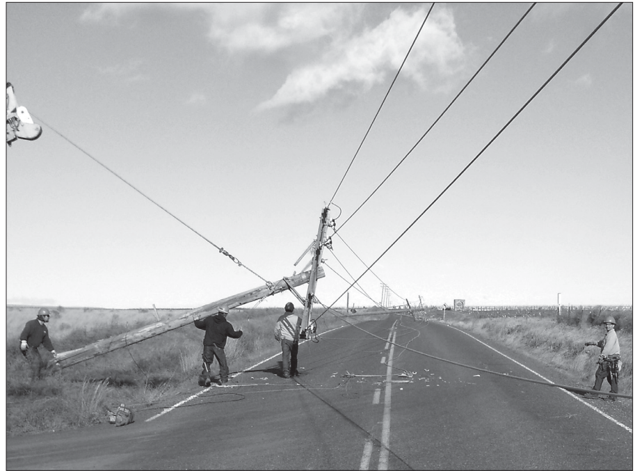
A storm in February 2008 knocked out power for approximately 12 hours while crews repaired multiple broken poles that snapped off in the severe wind.
