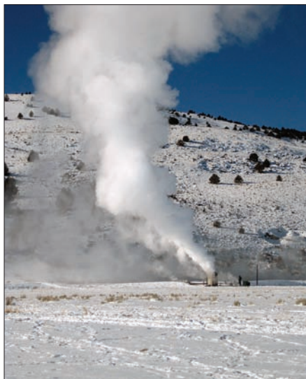
Above, steam rises from hot water underground through a well at the Paisley geothermal plant. Top, TBC workers unload the condenser unit, which was built in modules on a skid by Turbine Air System in Texas. TBC assembled the plant in Oregon.
