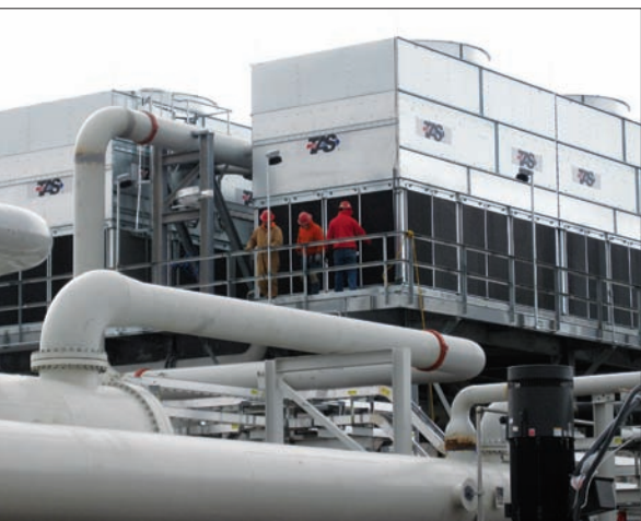
Colorado TBC crew members work on the cooling tower at the Surprise Valley Electrification Corp. geothermal plant in Paisley, Oregon.
