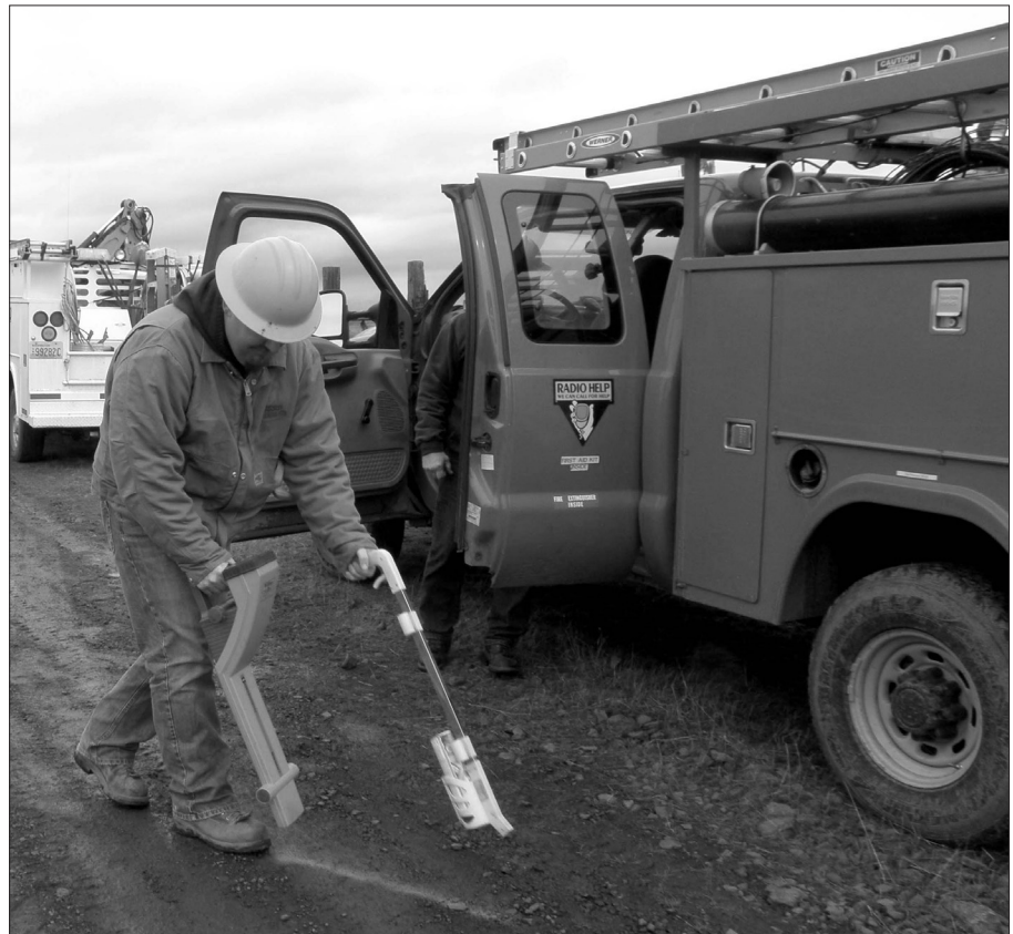
Travis Heilman demonstrates how an underground utility line is located and painted.
