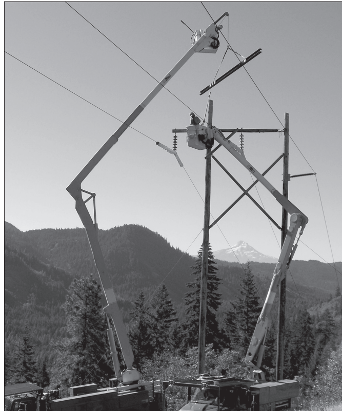
Repairs are made to the damaged structure on the Glenwood transmission line, while the line remains energized, or hot. Lake Howard flies the cross-arm in to Jeff Speelman and Todd Niva in the bucket.
