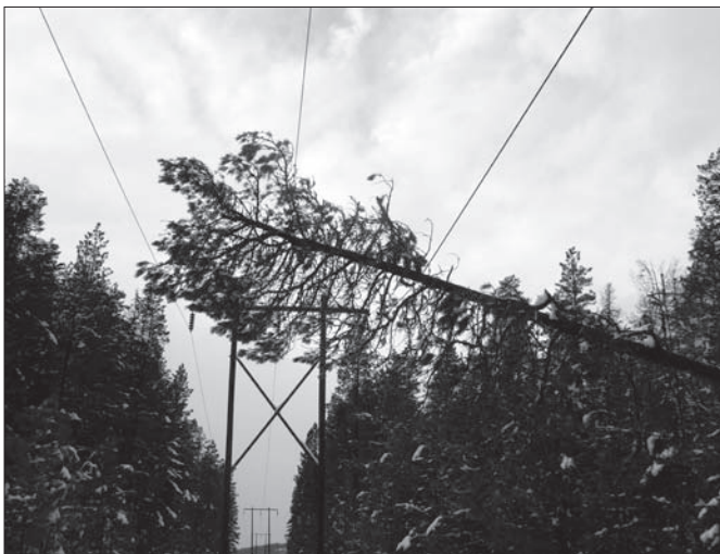
Lineworkers for Klickitat PUD untangled trees from the utility's Glenwood transmission lines after snow and ice in January 2012 brought down limbs and trees.
