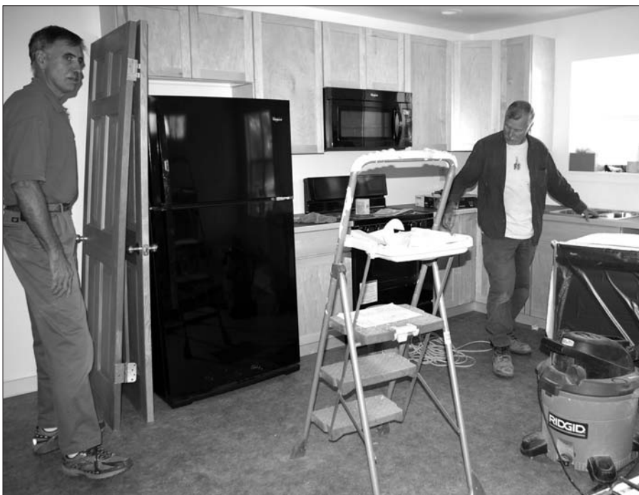
Volunteers Don Wanzek, left, and Stan Horack in the kitchen of an almost-complete Habitat for Humanity house in Lyle. The organization welcomes additional volunteers for other tasks in addition to construction.
