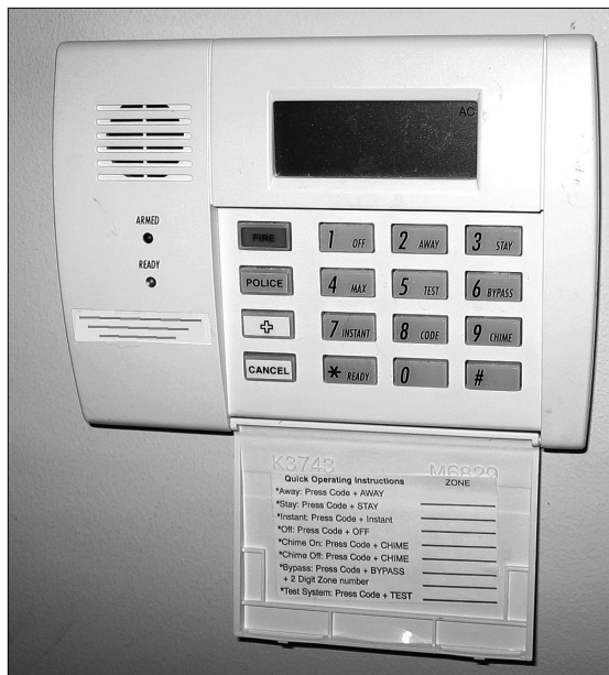
This wall-control module for a monitored security system has colored buttons for police, fire and health emergencies.
