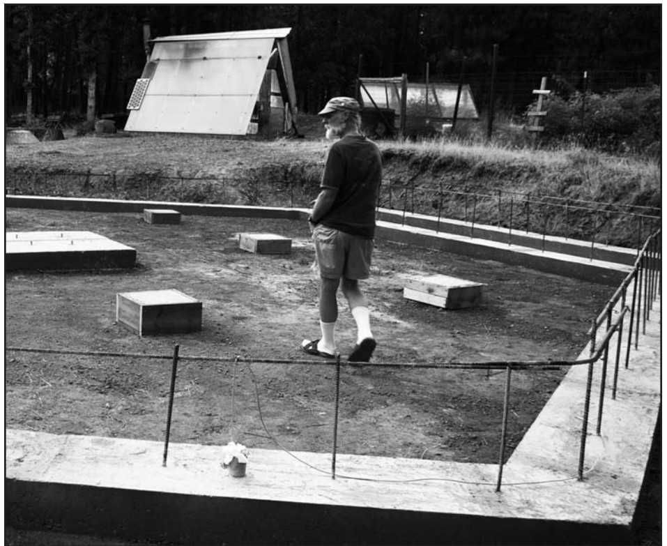
Above, longtime resident Tobiah Israel walks the foundation of the new eco-friendly house he and his wife are building. Below, Betty Long-Schleif walks to the round community building in the environmentally conscious Ponderosa Park community.
